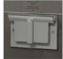
Duplex and/or GFI Outlets
