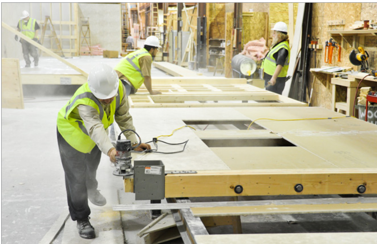
Construction of the modular classrooms at the Shelter Industries plant in Aldergrove, B.C.
