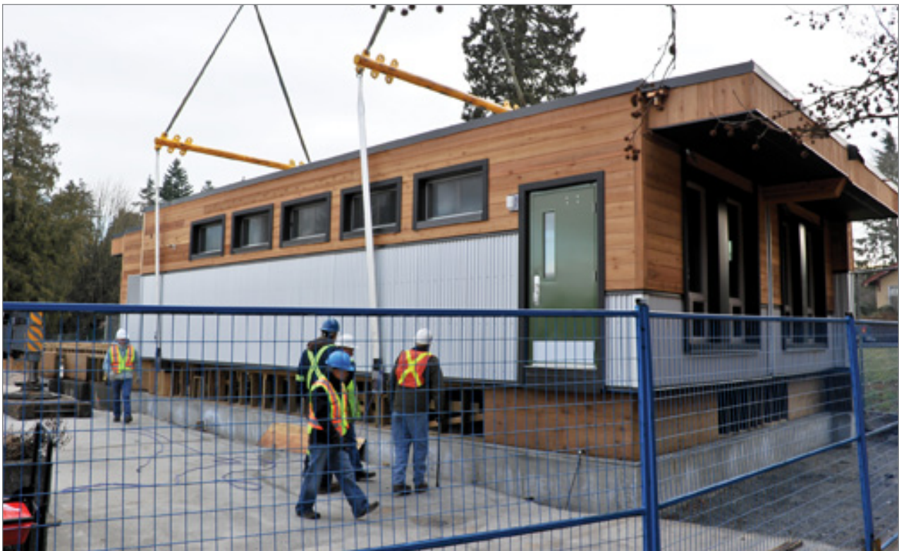
Workers complete the installation of the second half of a modular classroom at Herbert Spencer Elementary in New Westminster.
