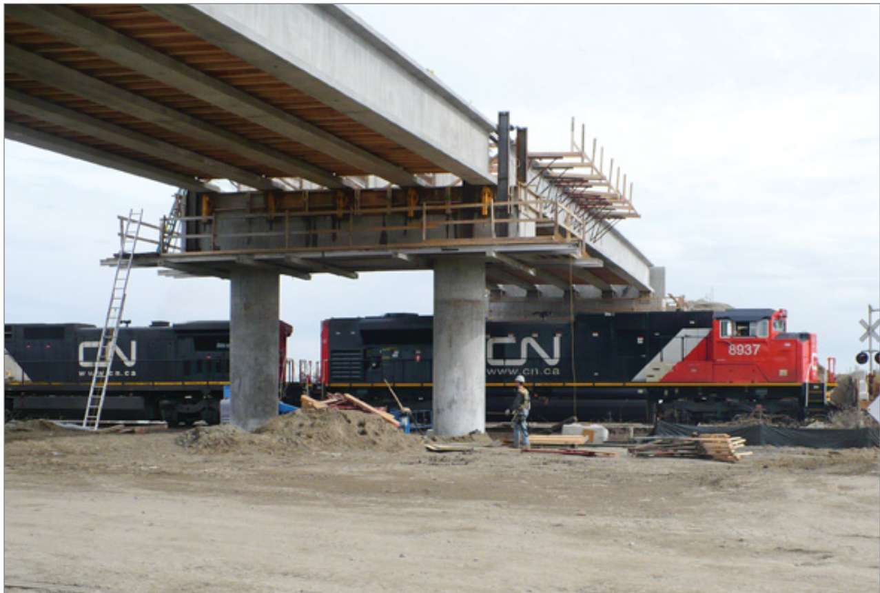
Construction of a new overpass to replace the existing at-grade rail crossing at 36th Avenue in Delta. The new overpass will allow continued access to farmland and local traffic flow.
